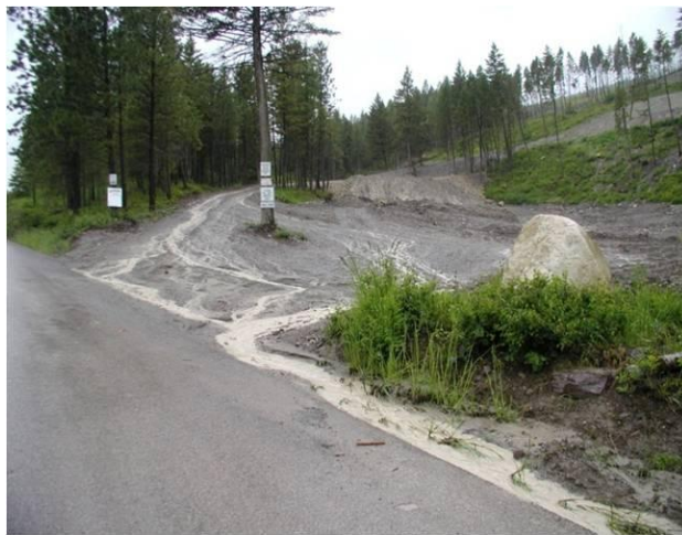
Figure 3. Erosion from Improper Development. Photo courtesy WLI
