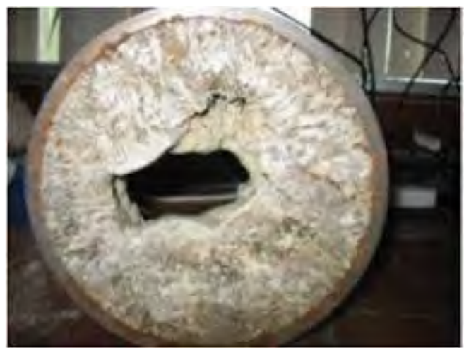
Struvite clogging pipes.
