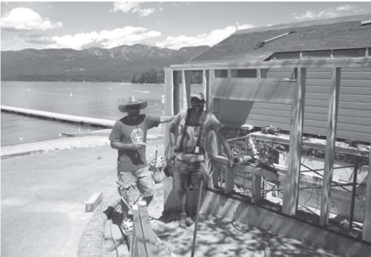
WLI is facilitating construction of the Whitefish Watercraft Inspection Station at City Beach with funding from the Joe & Cindy Gregory Family. Pictured are Nate Gibson and Chris Condiss from Trumble Creek Builders, the General Contractor.
