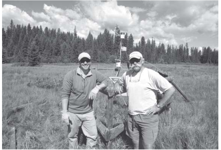
Volunteers Russell Chadwick and Chris Ruffatto pause after moving equipment out to the weather station to install new solar panels to power the bulk loading precipitation collectors.
